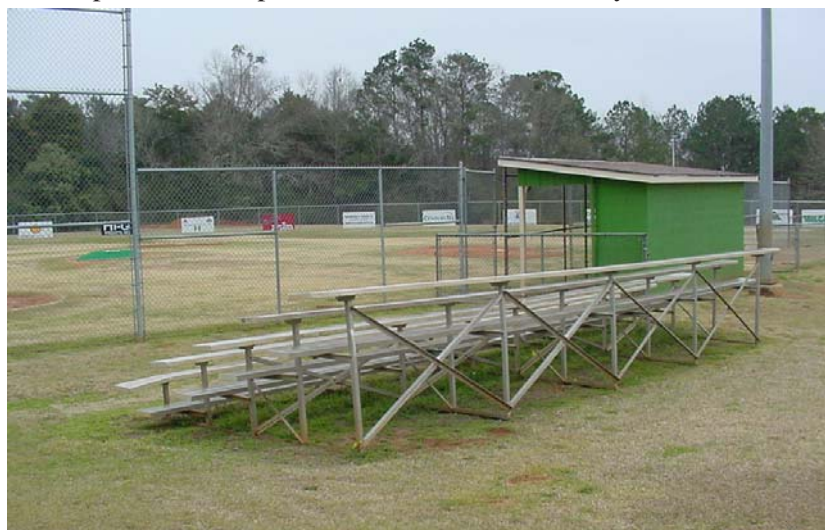
An all-too-common and extremely hazardous sight in many ball parks, these "old" bleachers are still in use without any guardrails.
